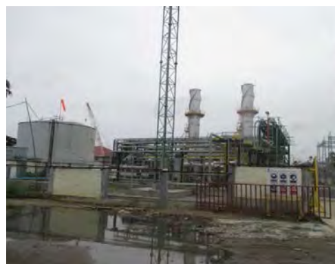
121MW GTCC Plant
