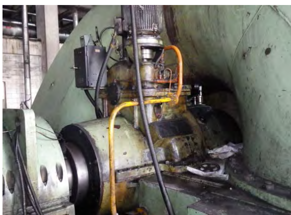
Turbine #2 Bearing House (frequent to vibration)
