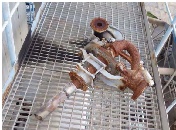
Unrestored broken Soot-blower
