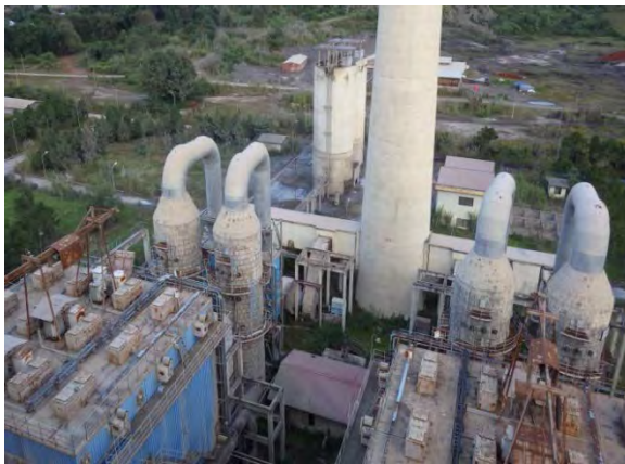
(from near side) Electrical precipitator, disabled FGD, Stack
