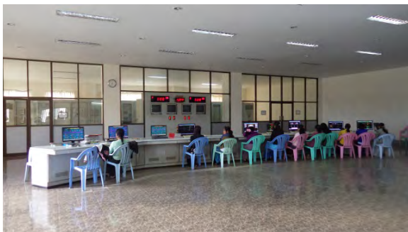
Central Control Room
