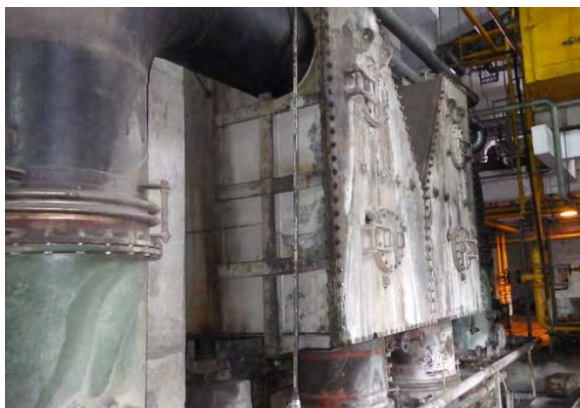
Condenser Water Box (difficult to open)
