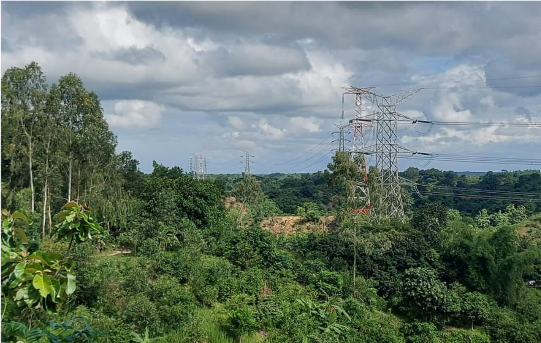
Figure 1: 400 kV TL line Through the Reserved Forest area
