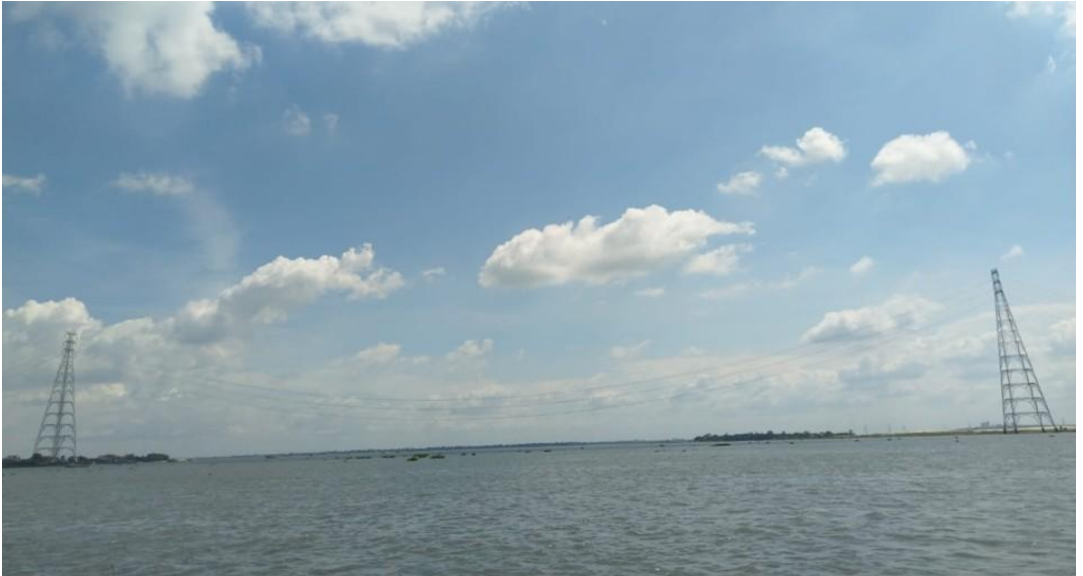
Figure 3: 400kV River Crossing Tower at Meghna River
