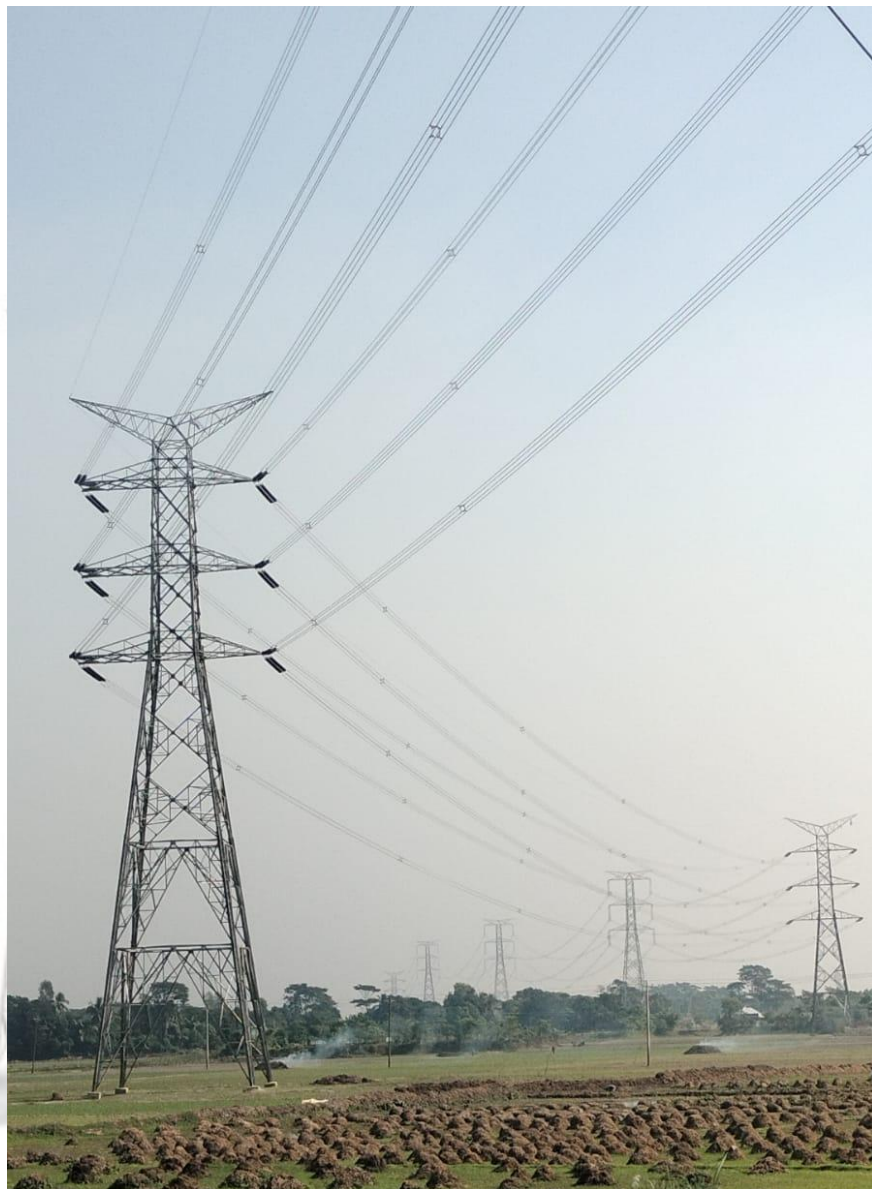
Figure 6: 400kV Transmission Line
