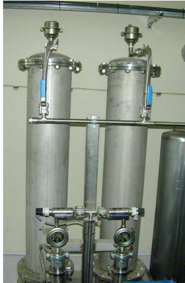
Ion Exchanger Chamber
