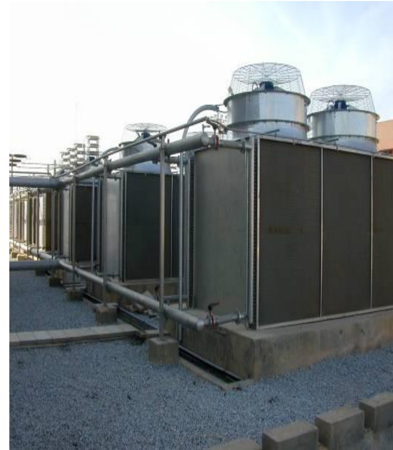
Valve cooling Tower
