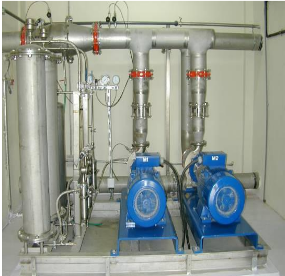
Valve Cooling Pump
