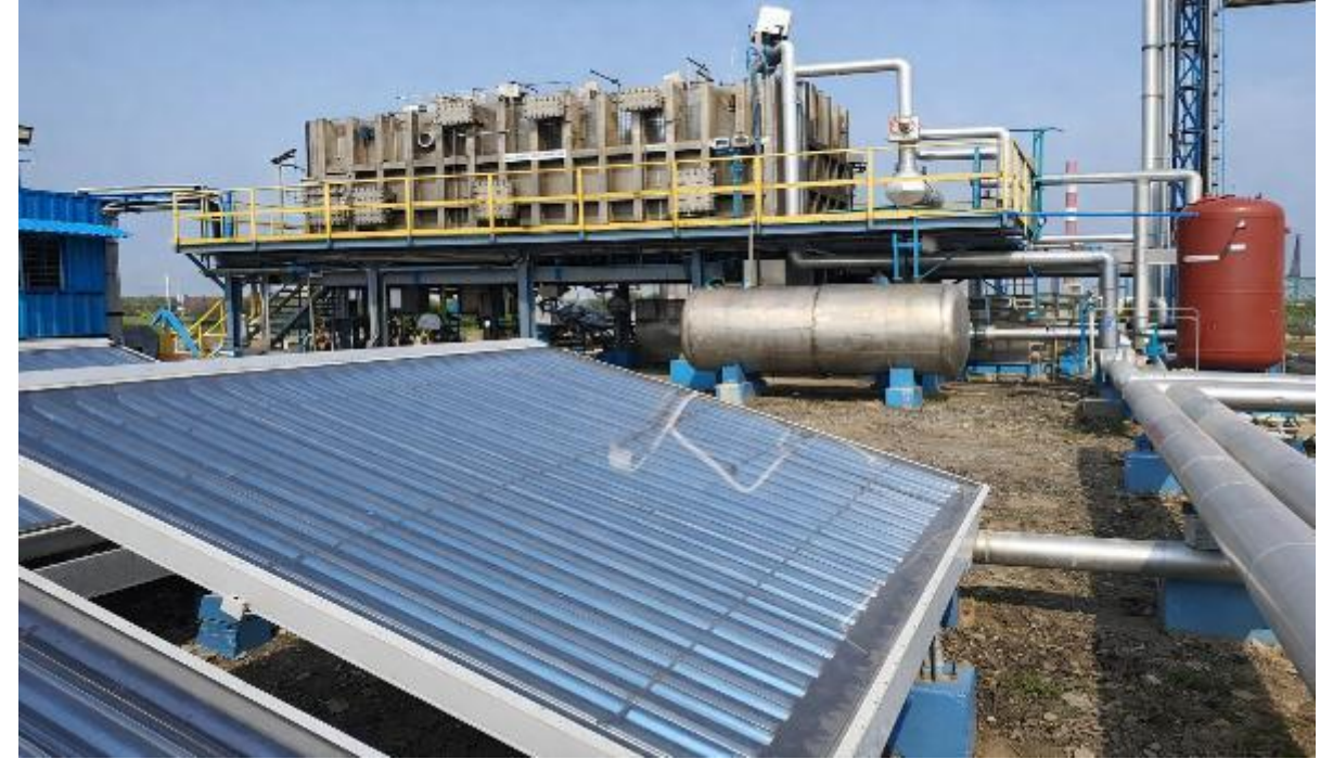
Using Solar Thermal for Desalination Plant at NTPC Vallur Under Operation
