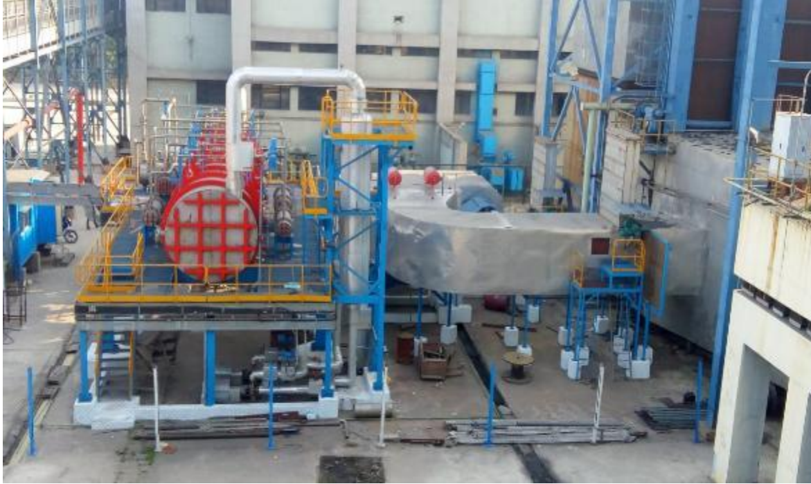
Using Waste Flue Gas from Coal Based Plant 120 TPD Desalination Plant at NTPC Simhadri Under Operation
